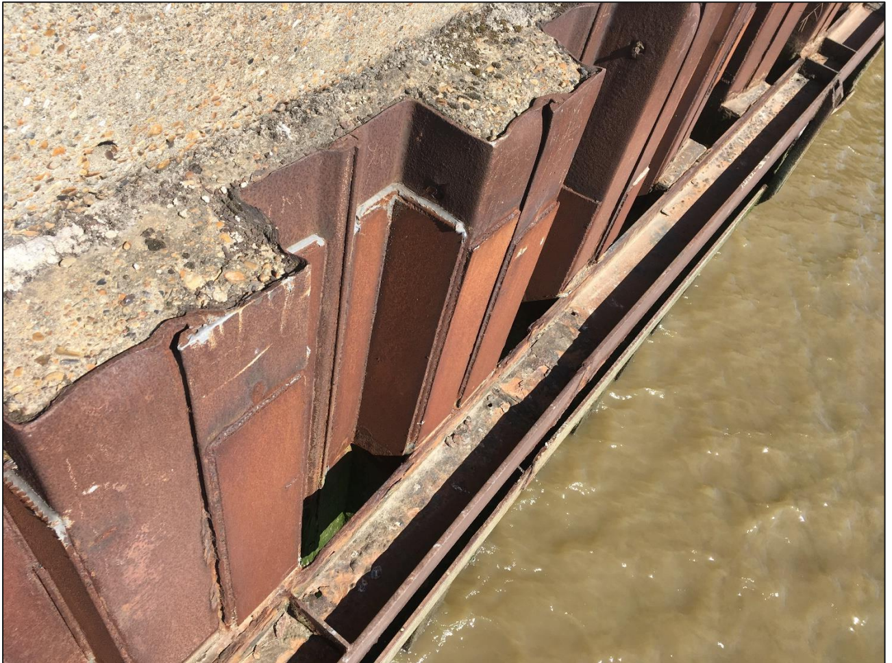
Figure 3.1: Typical photograph of upper level of river wall, showing steel plate repairs to sheet piling, taken from the land side of the river wall
