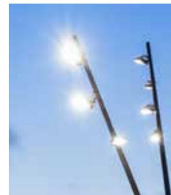
Pole mounted lighting
