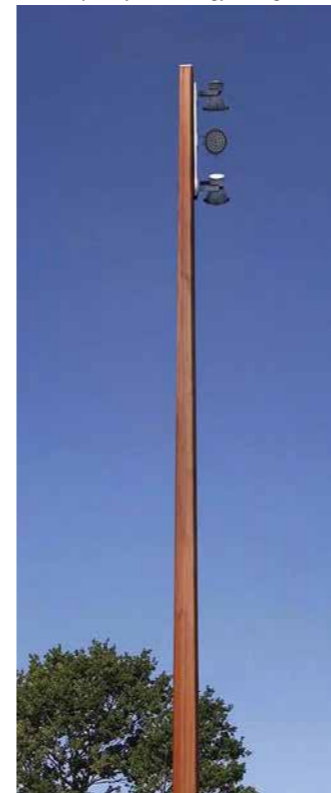
Timber pole lamp-posts to soft areas
