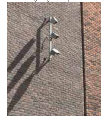
Façade mounted street lighting
