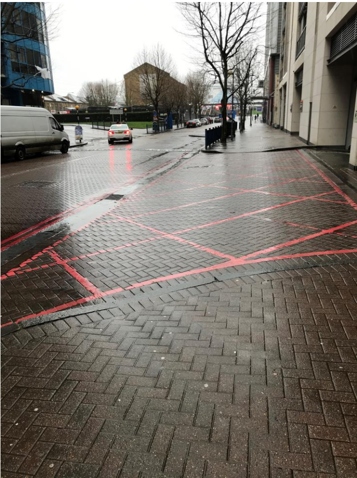
Very wide bellmouth/crossover for car park access
