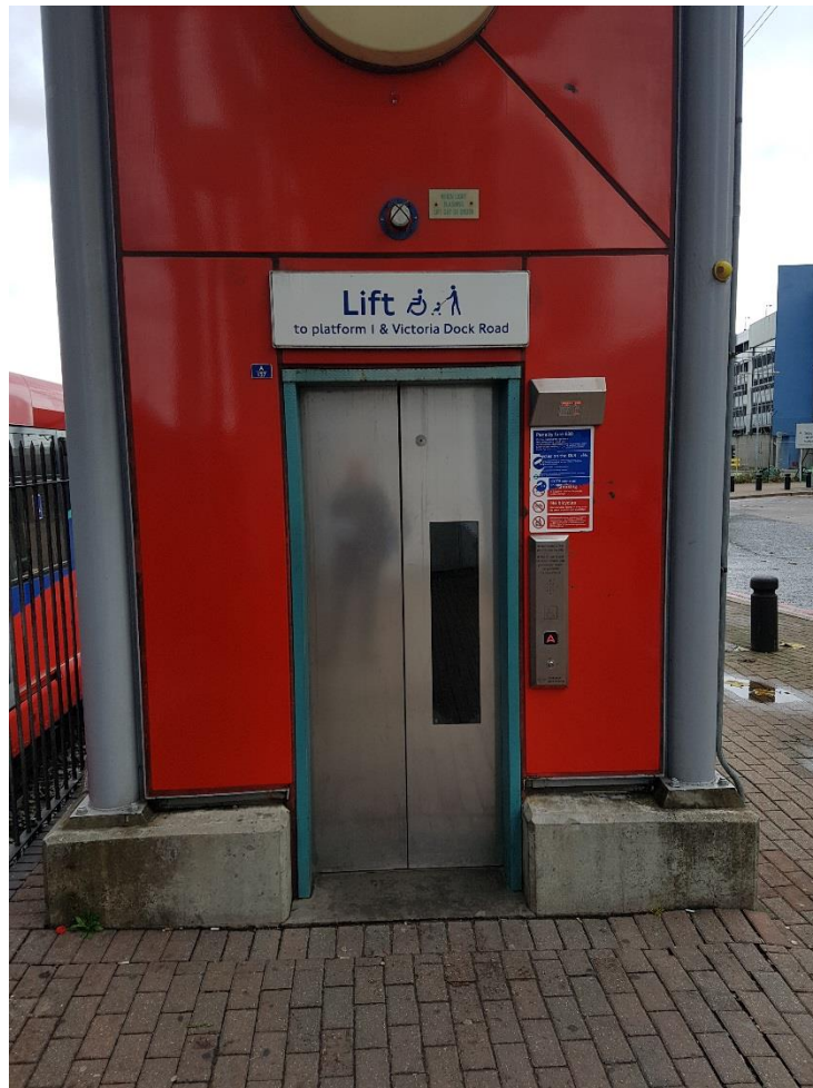
Figure 19. Lift at Royal Victoria Station
