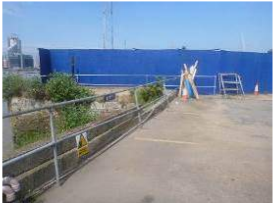
Figure 26 - Impact damage to concrete parapet and possible settlement behind the frontage
