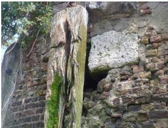
Figure 31 - Voided masonry behind remains of timber fender
