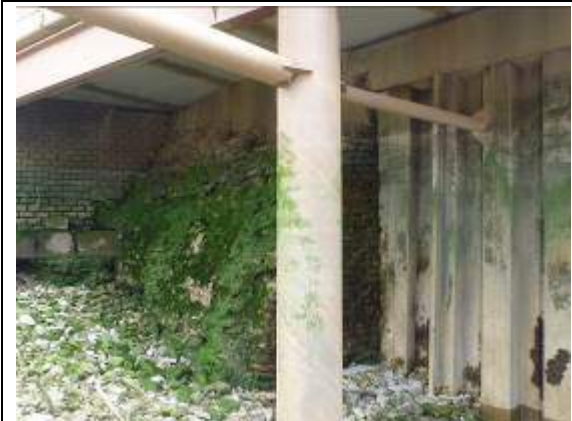
Figure 5 - Concrete bagwork section with steel frame for spoil transfer hopper in foreground
