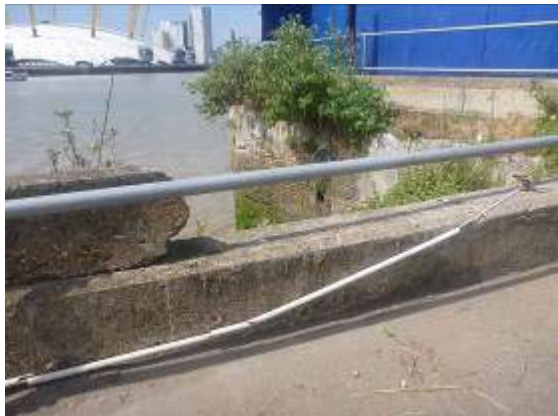
Figure 28 - Missing section of raised concrete parapet
