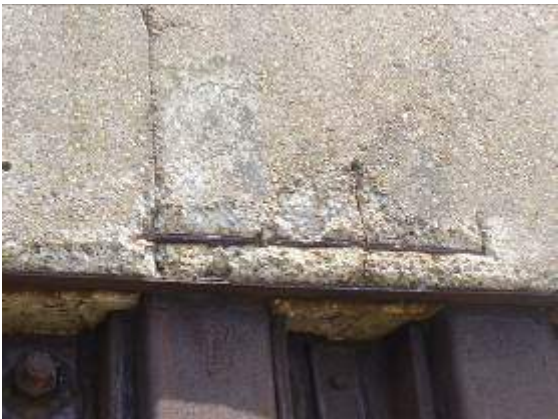
Figure 60 - Spalling to soffit of concrete capping beam with exposed corroded steel reinforcement
