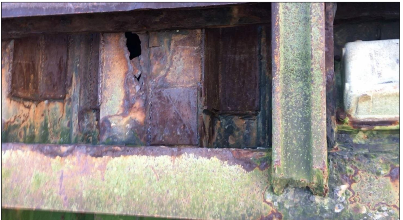
Figure 3-2: Location where patch repair to perforation in steel sheet piling has been missed
