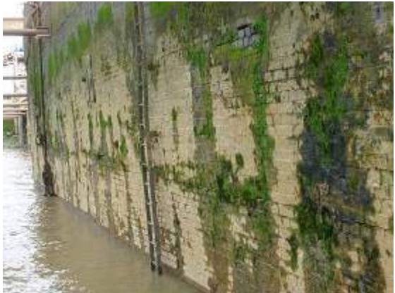
Figure 12 - View of misalignment and bulging in wall
