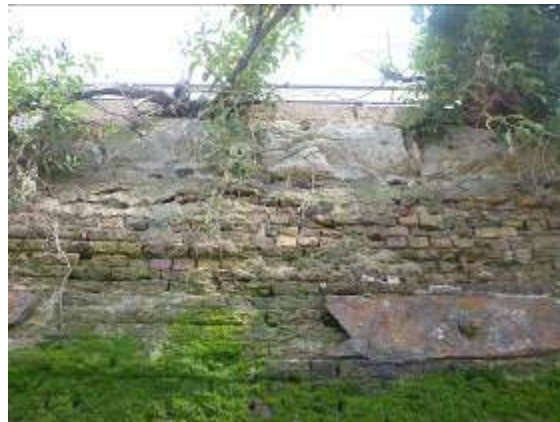
Figure 30 – View of eroded masonry wall with concrete parapet and remnants of steel waling beam.
