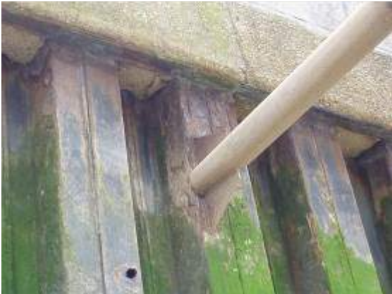
Figure 18 - Welded connection to brace hopper support frame. Elevated corrosion of piles around connection evident
