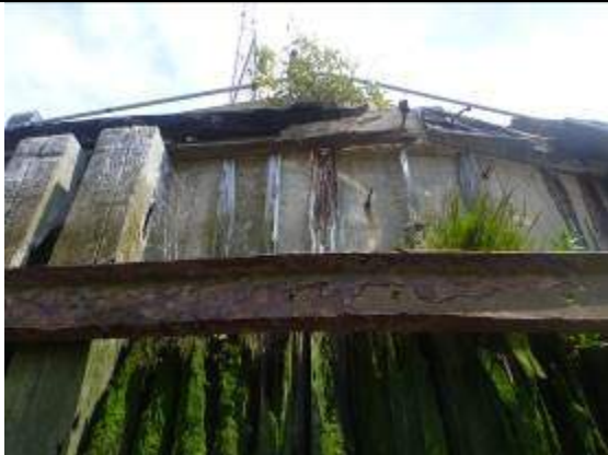
Figure 20 - Corroded steel restraint channel which is separating from the wall
