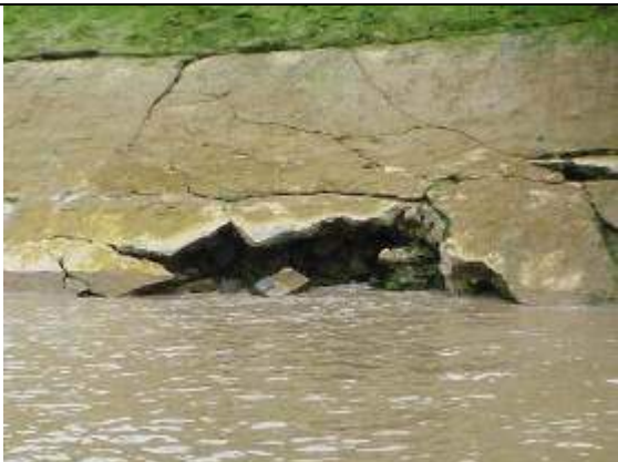
Figure 25 - Void in concrete apron
