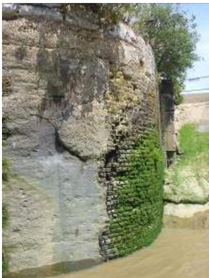
Figure 22 - Large vertical crack in masonry section
