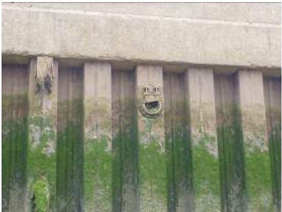
Figure 4 - Broken flap valve on sheet pile wall
