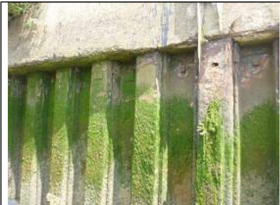
Figure 57 – Splash zone corrosion and erosion of soffit of the concrete capping beam
