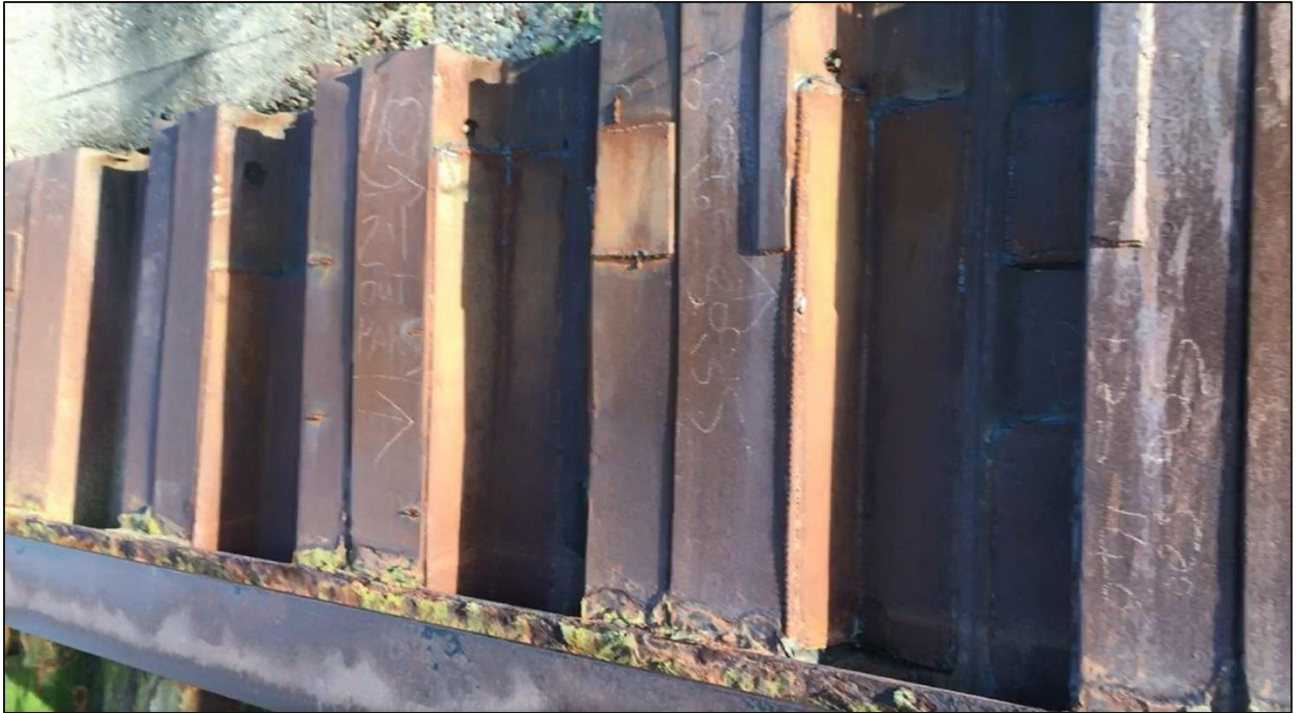
Figure 3-1: Typical photograph of upper level of river wall, showing steel plate repairs to sheet piling
