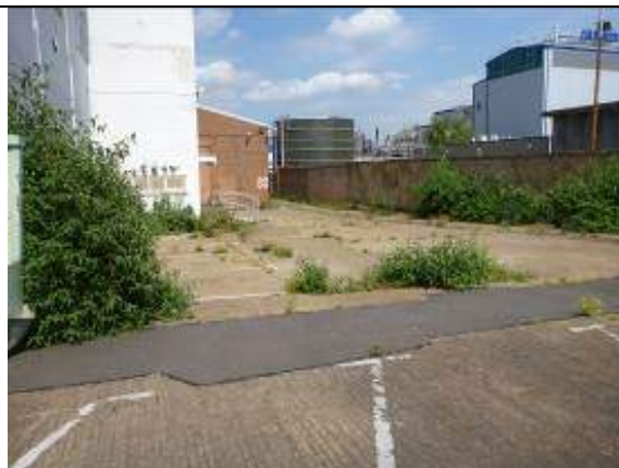
Figure 68 - Cracked and uneven surfacing behind the frontage
