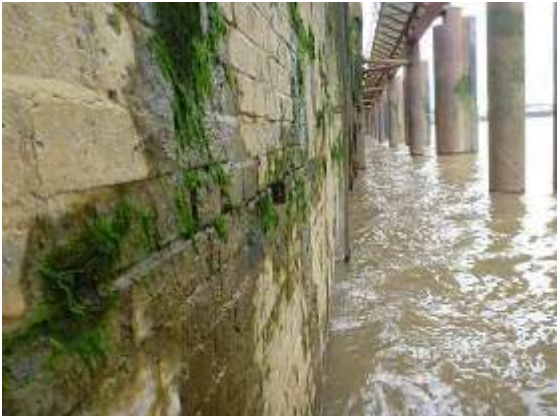
Figure 13 - View of horizontal crack in bed joints mid-height between bed level and anchor height
