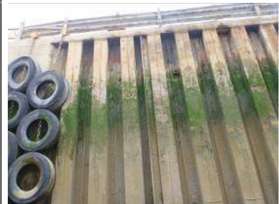
Figure 56 - Perished waling bolts
