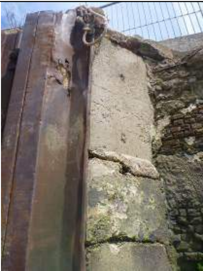
Figure 34 – Damage to concrete interface between sheet pile wall and downstream adjacent masonry wall
