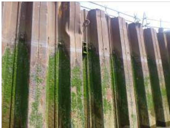
Figure 42 - Impact damage to steel sheet piles
