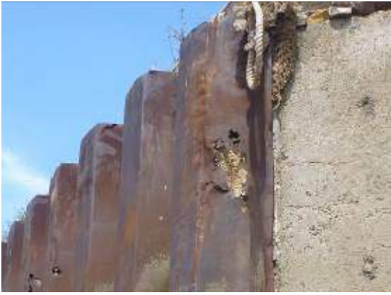
Figure 36 – Full-thickness corrosion at the downstream extent of the frontage
