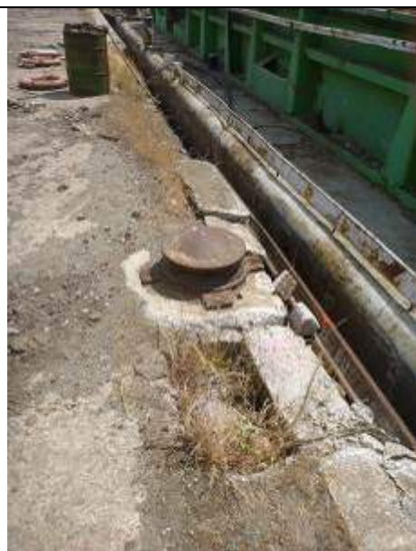
Figure 51 – Damage to coping adjacent to mooring bollard
