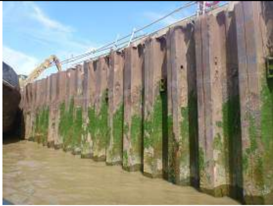
Figure 40 - Steel sheet pile wall with crumple damage to the top of the piles
