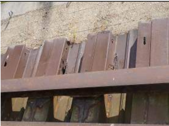
Figure 64 - Full depth corrosion of steel sheet piles with voids in the concrete back fill
