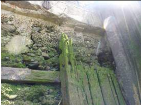
Figure 75 - Timber wall and voids in concrete at intersection with steel sheet piling
