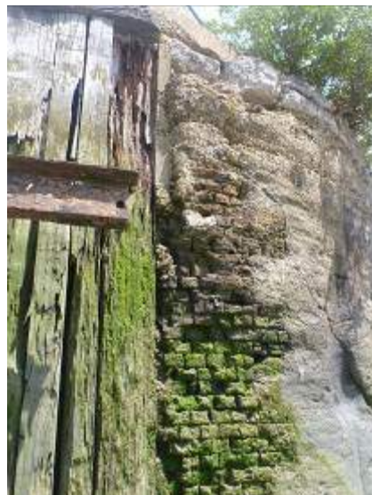
Figure 23 - Loss of pointing in masonry section, together with rotten timber cladding
