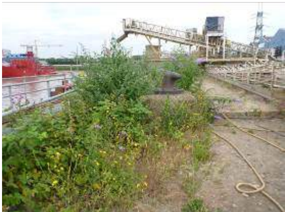
Figure 19 - Vegetation growth behind the raised flood wall
