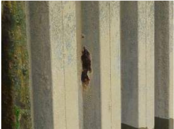
Figure 17 - Localised corrosion, possible Accelerated Low Water Corrosion
