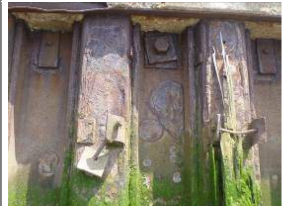
Figure 59 - Accelerated corrosion of steel sheet piles at welded connections
