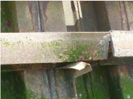
Figure 66 - Impact damage to waling beam
