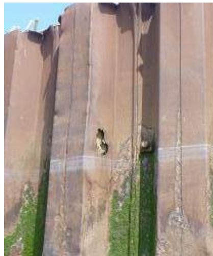
Figure 43 - Localised full-thickness corrosion to sheet piles
