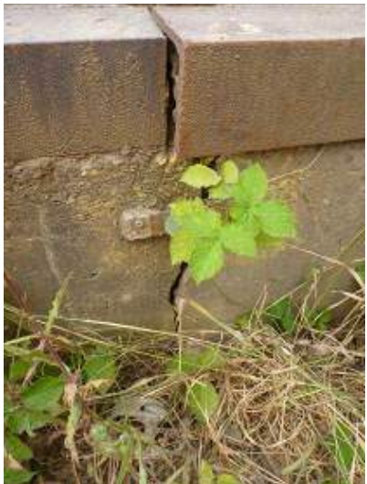
Figure 14 - Crack in concrete parapet with crack monitoring plates
