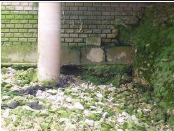
Figure 6 - Blockwork wall frontage with localised erosion at toe of wall
