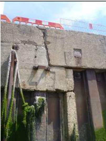
Figure 58 – View of break in construction – joint in capping beam and concrete “plug” in place of pile below joint
