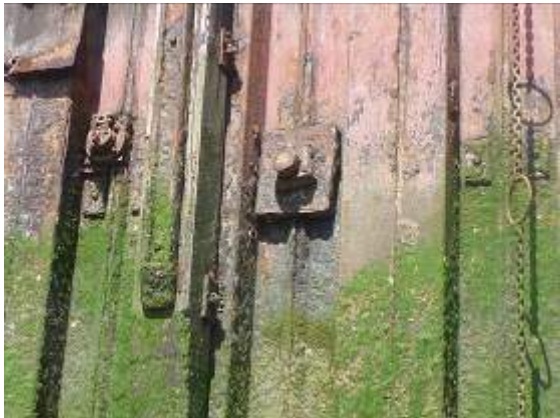
Figure 72 - Corroded waling and anchor bolts
