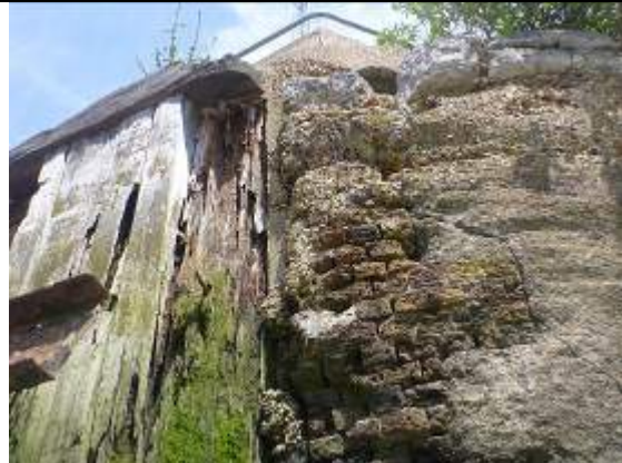
Figure 21 - Interface between exposed masonry sections and timber clad section. Masonry is badly eroded or missing. Large repairs using (sprayed) concrete
