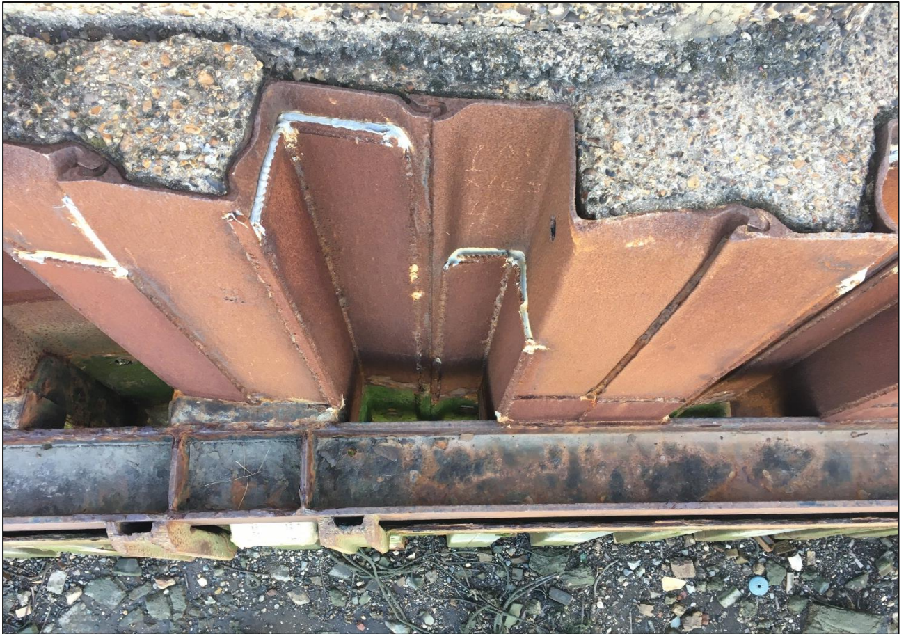
Figure 3.1: Typical photograph of upper level of river wall, showing steel plate repairs to sheet piling, taken from the land side of the river wall
