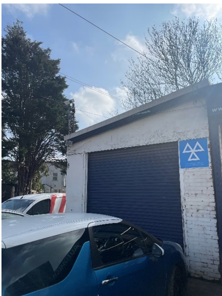
Figure 3-1 Roller Shutter Doors
