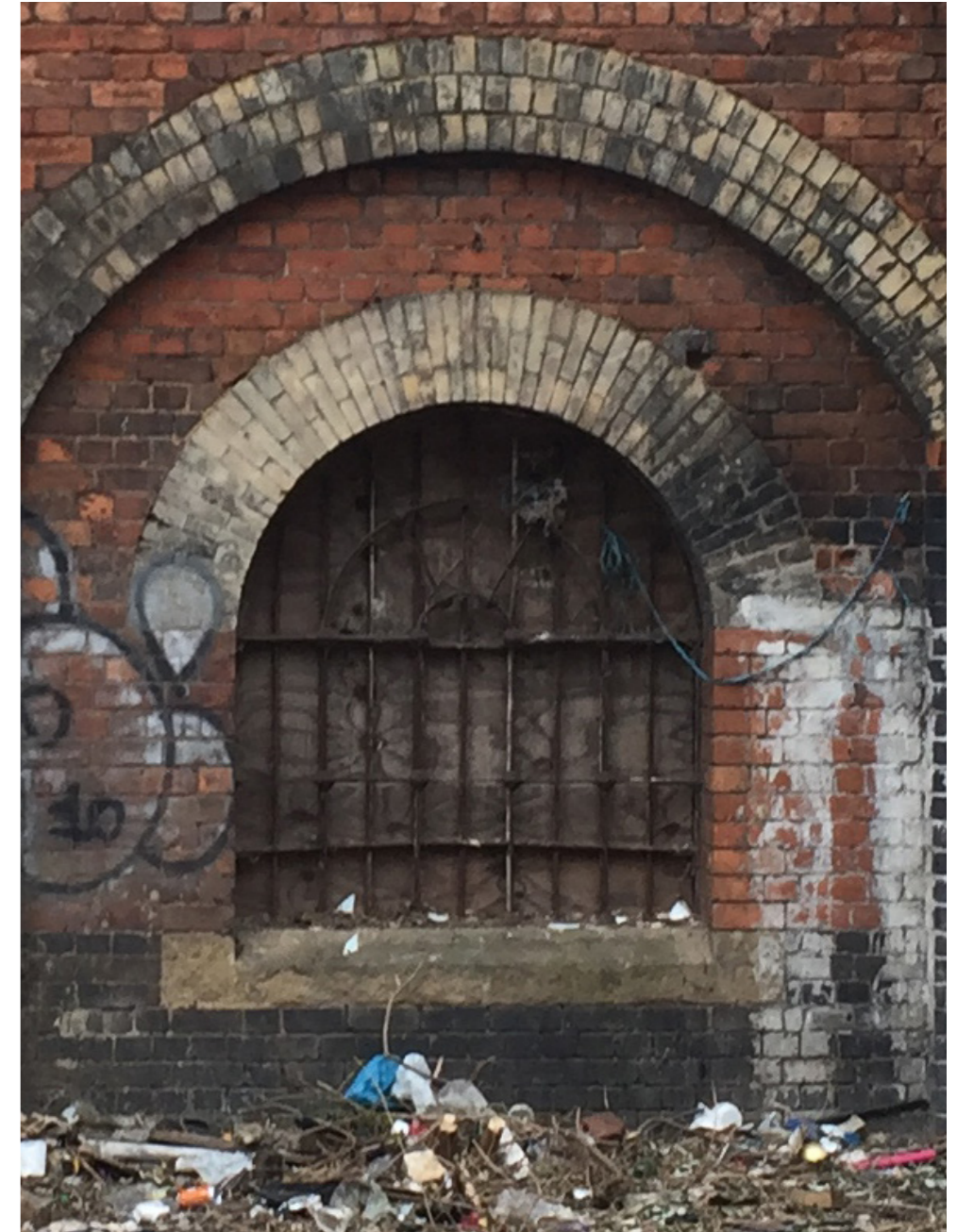
Station Wall, example of surviving cast iron window frames, to be retained.
