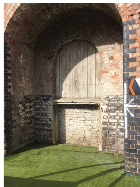
Photograph showing the rear of the wall, showing the depth of the arches
