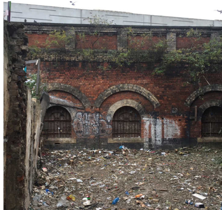
Station Wall behind the Weavers Cottages. The arches retain some cast iron window frames, which will be set aside for reuse.
