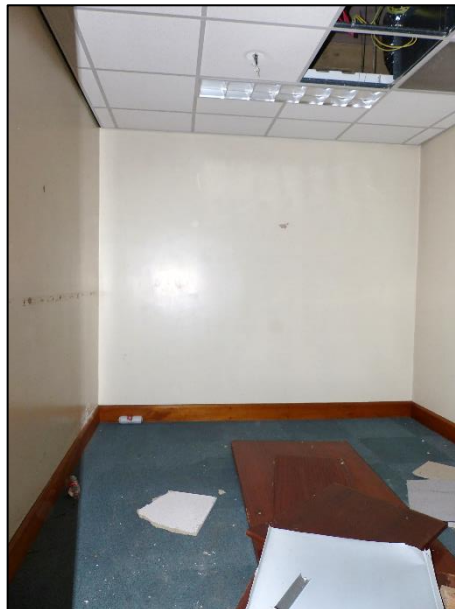
Fig 72 An example of the interview rooms/office to the west end of the high security section, looking south P1400175
