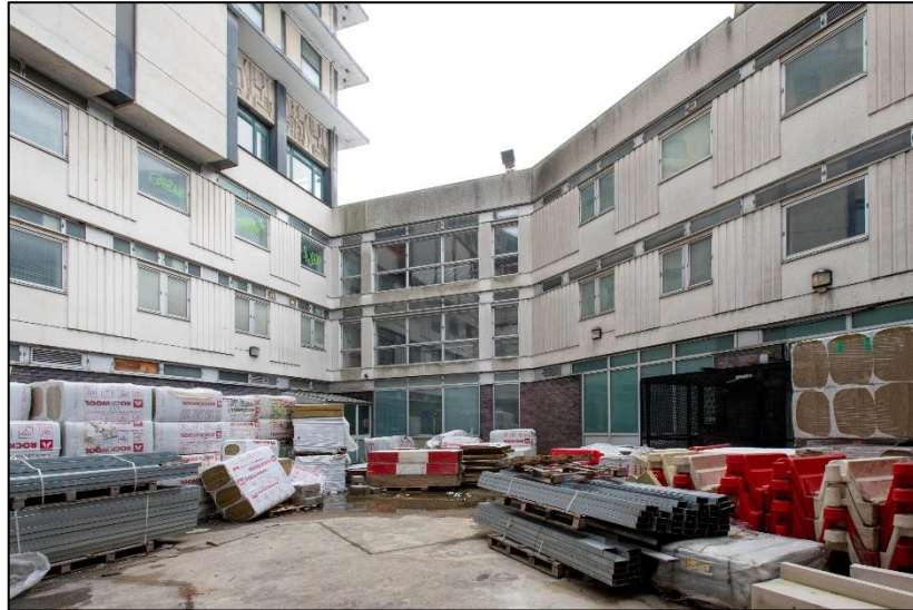
Fig 30 A general view of the pentagonal yard, looking south-east (centre); the caged access (in black) to the custody suite is visible to the right side of the image (A. Chopping) 035322007
