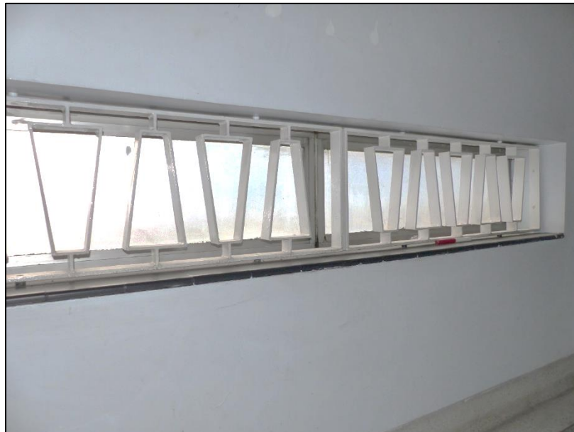
Fig 117 The wrought iron grill to the landing window between the ground and first floors, looking south-west P1400336
