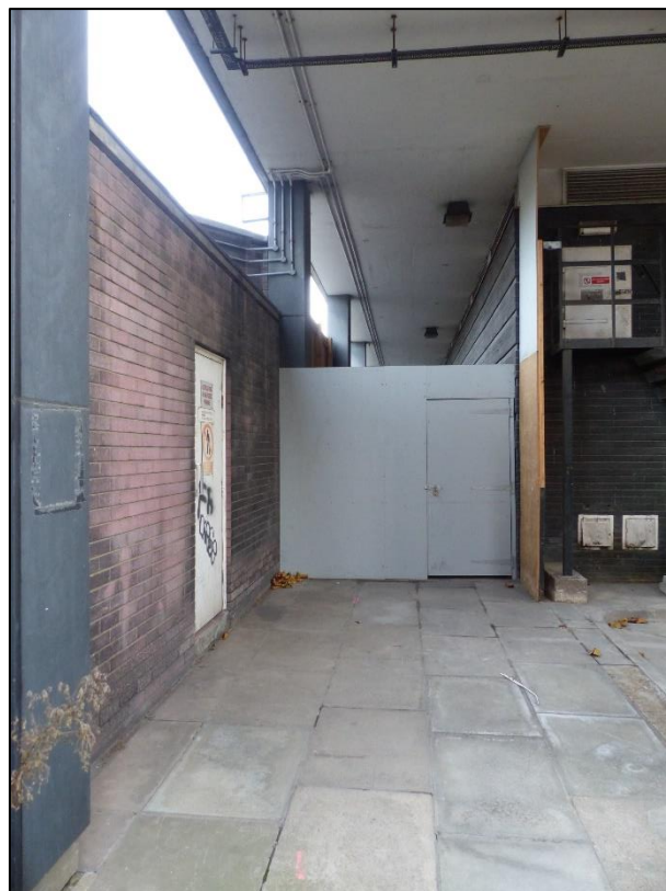
Fig 24 The hoarding blocking the open walkway to the north-east elevation, looking south P1400298
