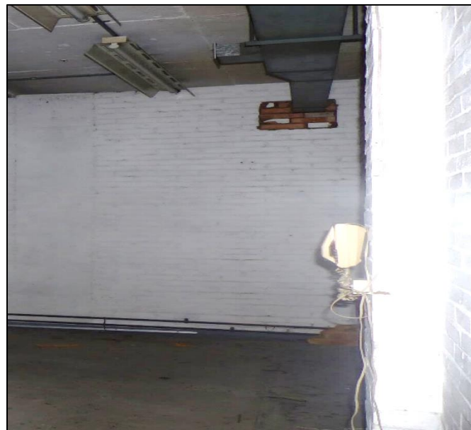
Fig 45 General view of a storage room in the basement, looking south-east P1330273
