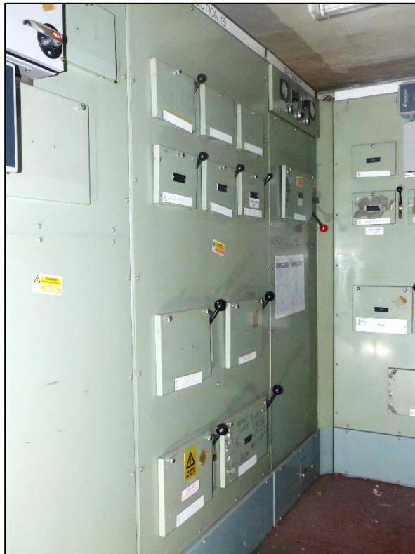
Fig 43 The electric controls for the station (Electric Intake room) in the basement, looking south-east P1330262
