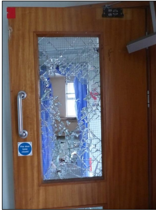
Fig 9 Damaged door on one the 7th floor of the Section House, possibly made during the eviction P1330227
