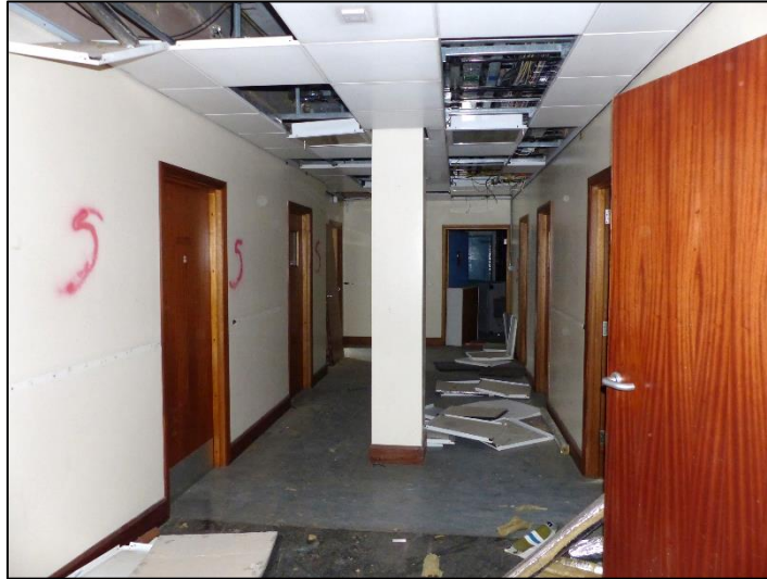
Fig 69 The offices and interview rooms to the high security section, looking east P1400201
