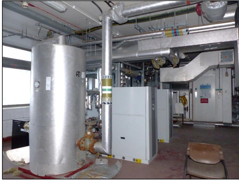
Fig 126 An example of the plant seen to the upper storeys of the eight-storey tower block, looking north-east P1400351
