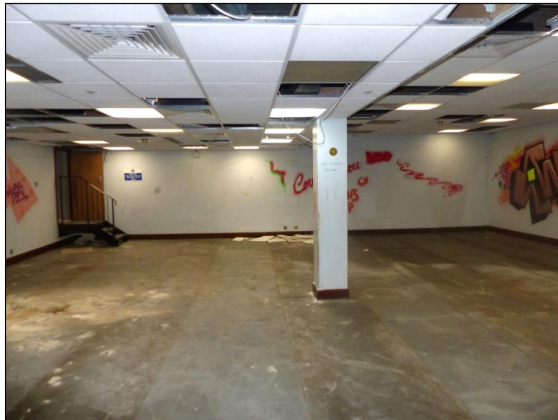
Fig 41 The former Parade Room in the basement, looking north-east from the access corridor stairs; note the door and stairs to the electric intake room (left side of the image) P1330254
