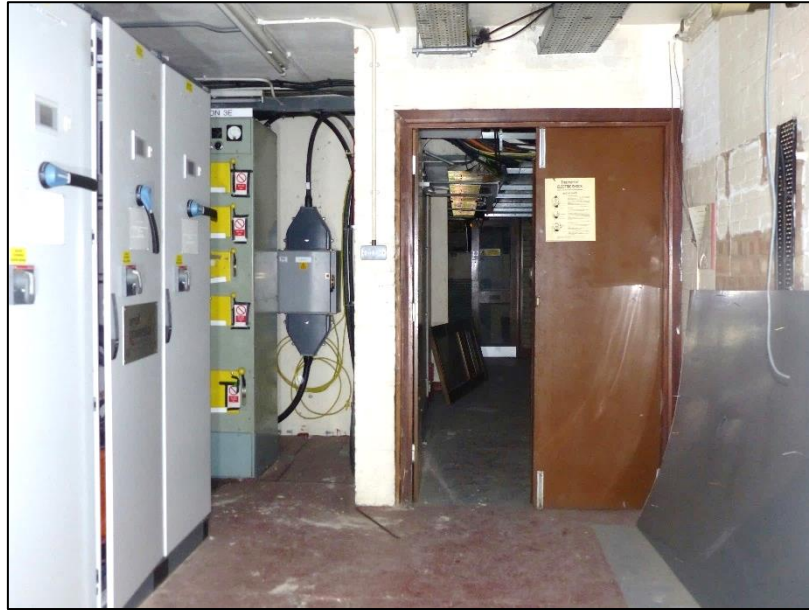
Fig 42 The Electric Intake room in the basement showing access to the storage areas and rooms to the north, looking south-west P1330260
