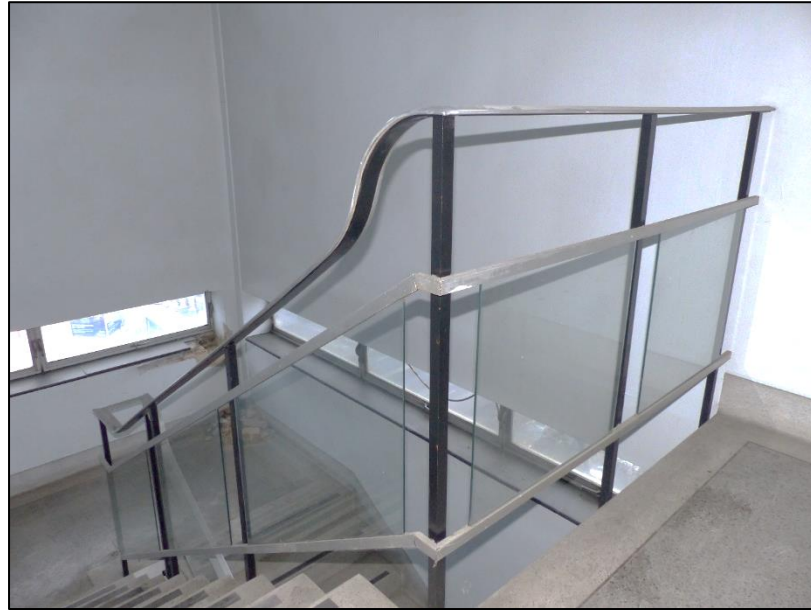
Fig 116 The stairs to the west side of the eight-storey block, looking south-west P1400353
