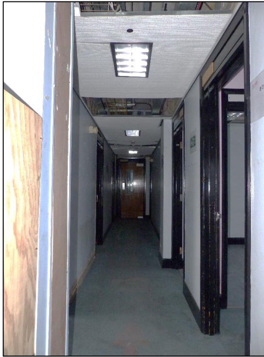
Fig 120 A typical corridor seen on the second floor of the eight-storey block, looking east P1400341
