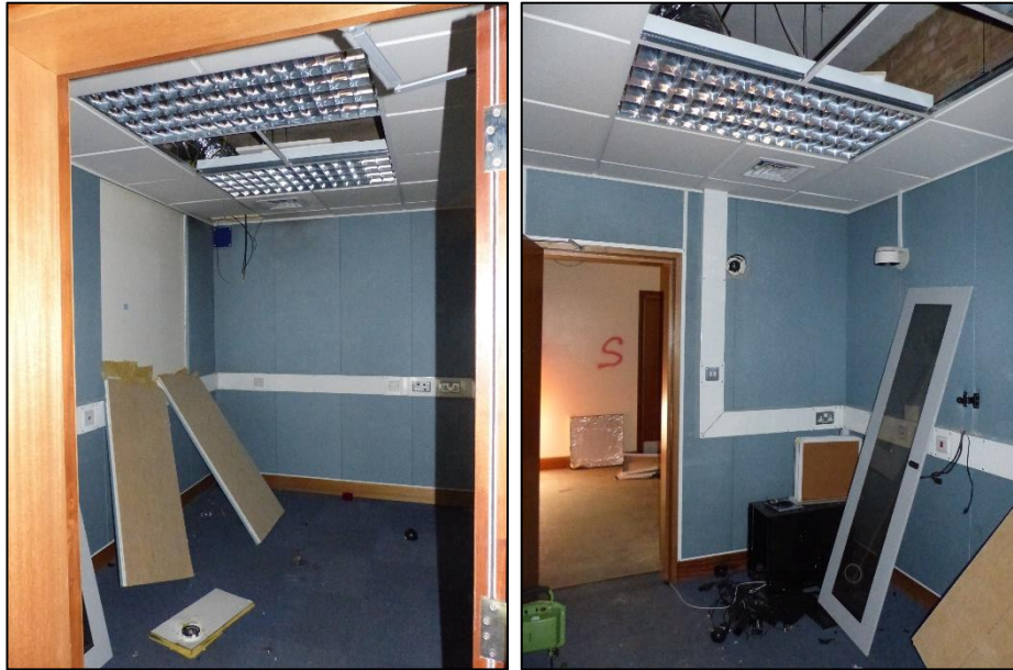
Fig 71 An example of a soundproof room, looking south and north respectively P1400208 and P1400209
