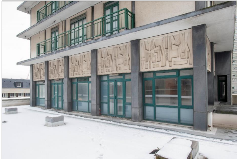
Fig 29 North-west exterior elevation to the third floor as seen from the roof (A. Chopping) 035322030
