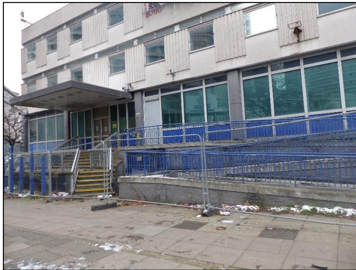
Fig 21 The concrete ramp to the east of the main public entrance, looking north-west P1330198
