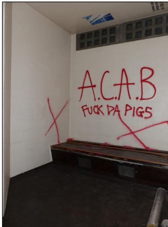
Fig 6 Graffiti against the cops on a holding cell wall at the ground floor, looking north-west P1400165
