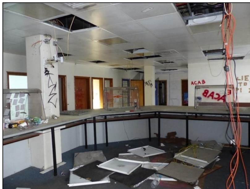
Fig 8 Ground floor custody counter with squatters' leftovers and ceiling tile damage, looking south-west P1400153
