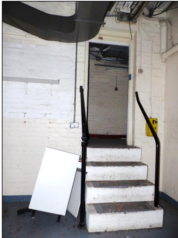
Fig 44 A storage room and good example of the changing levels and earlier brickwork within the basement, looking south-west P1330266
