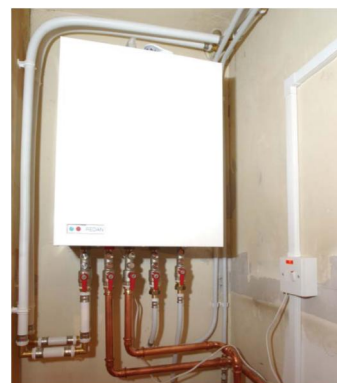
Figure 15: A heat exchanger inside one of the flats connected to the Aberdeen district heating network (Source: Aberdeen City Council: a case study of community heating CE65, Energy Saving Trust, 2003)
