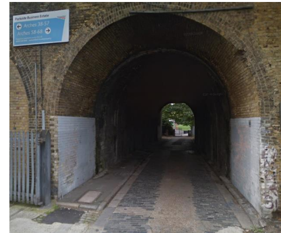
Figure 21 Archway area looking south west prior to resurfacing. Ground scarring indicates location on UKPN cables
