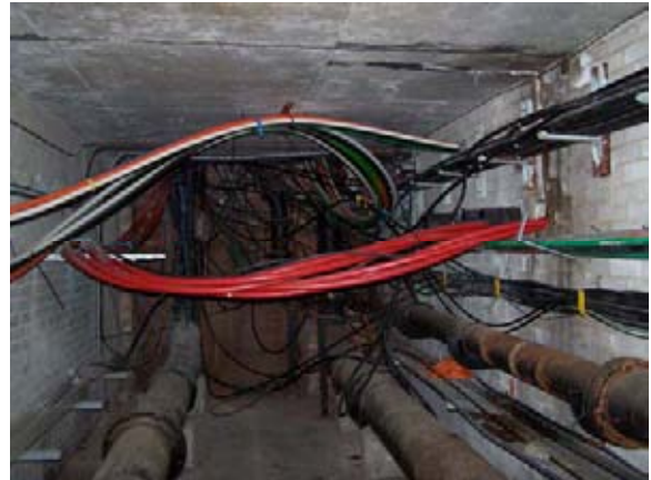
A further take off point. The triplex red sheathed cables running left to right are high voltage, probably 11kV.
