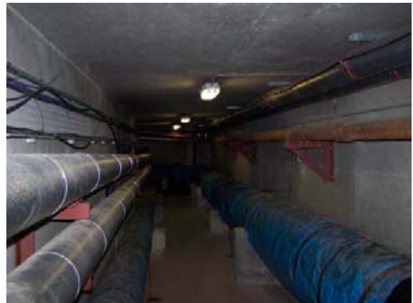
Organised pipe and cable runs: large pipes
