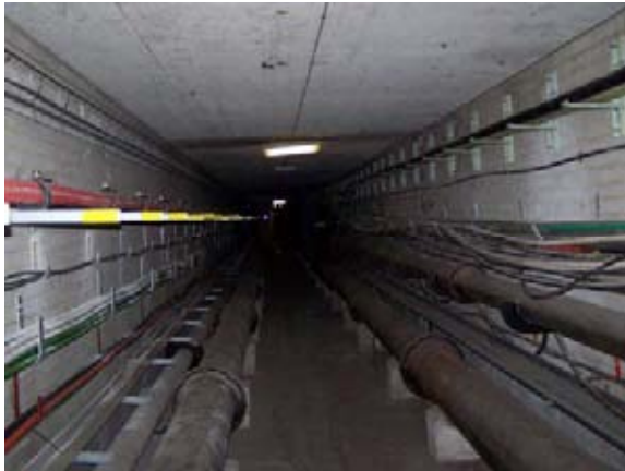
Well organised pipe and cable runs. HV cables and LV cables to the left, uninsulated pipes at low level and comms cables to right
