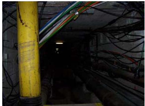
Illustration of current lighting. Vertical pipe would appear to be a gas service. Untidy cabling to the right.
