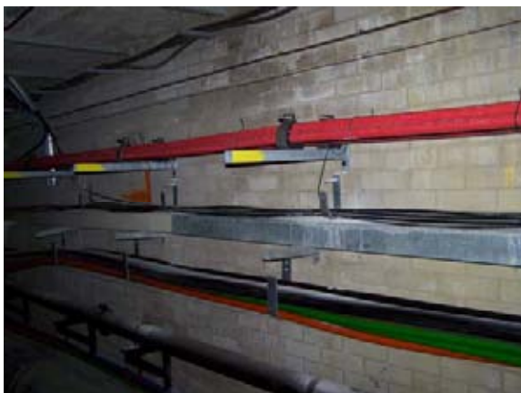
Cable supports: HV cables at top, comms middle, LV lowest. No labels apparent.
