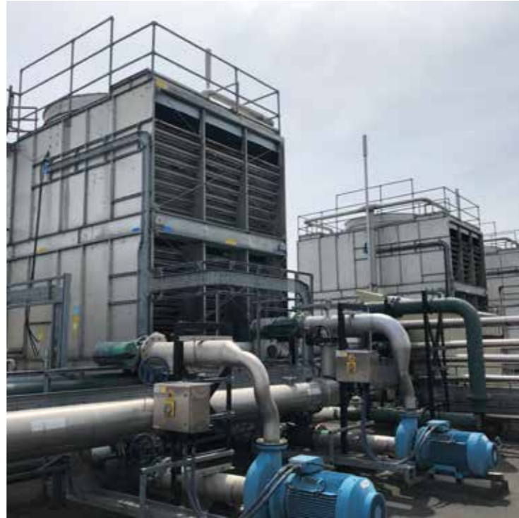
Air conditioners at roof of energy centre
