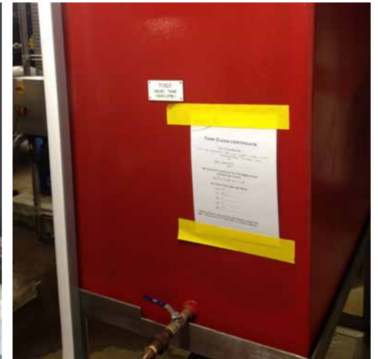
Decommissioned diesel tank in Production Office basement
