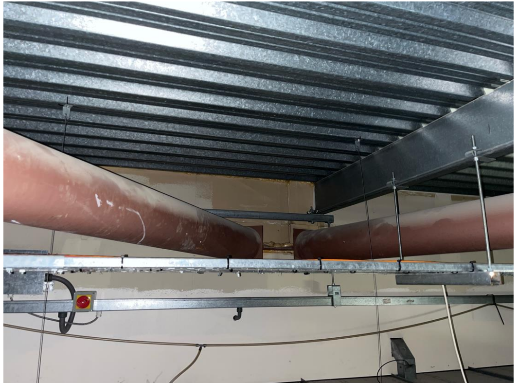
Figure 4 - Steel structure found in roof space of entertainment building
