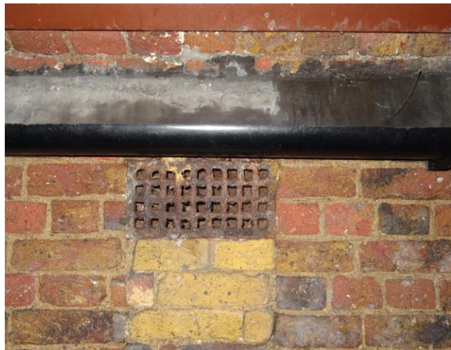
Photograph 9: Small dark voids in the piers of the tunnels of Area B which had a metal grill.
