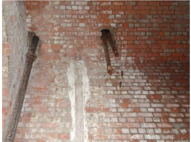
Photograph 4: Area A gaps between pipework and brickwork.
