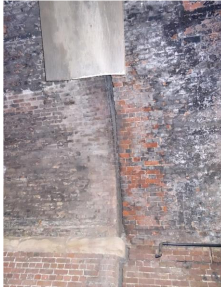
Photograph 10: Large gaps between tunnel section joins in Area B.
