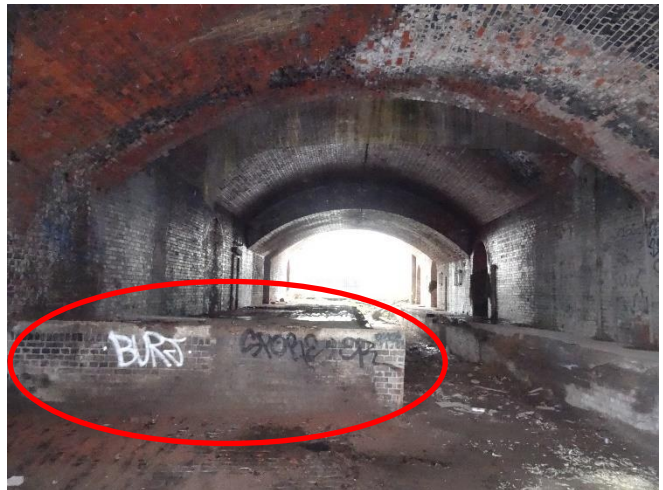
Photograph 2: BPZ1 raised section (circled in red) with hole leading to underground archways / cellar
