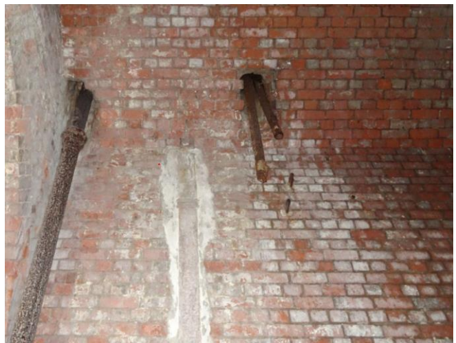
Photograph 4: BPZ1 gaps between pipework and brickwork.
