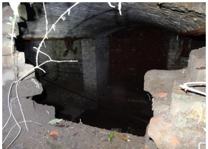
Photograph 3: BPZ1 underground cellar / archway seen through a hole beneath raised section within a tunnel.
