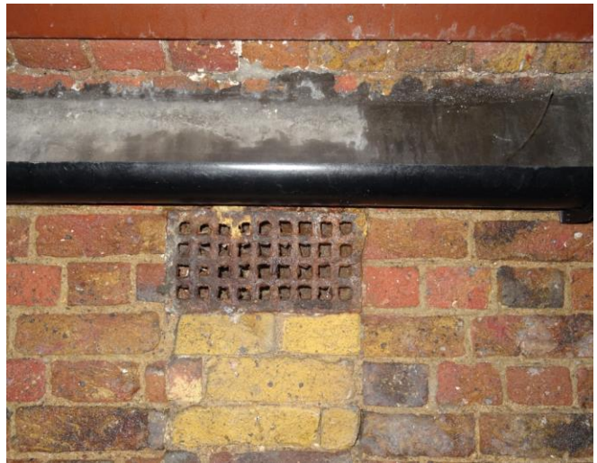
Photograph 8: Small dark voids in the piers of the tunnels of BPZ2 which had a metal grill.
