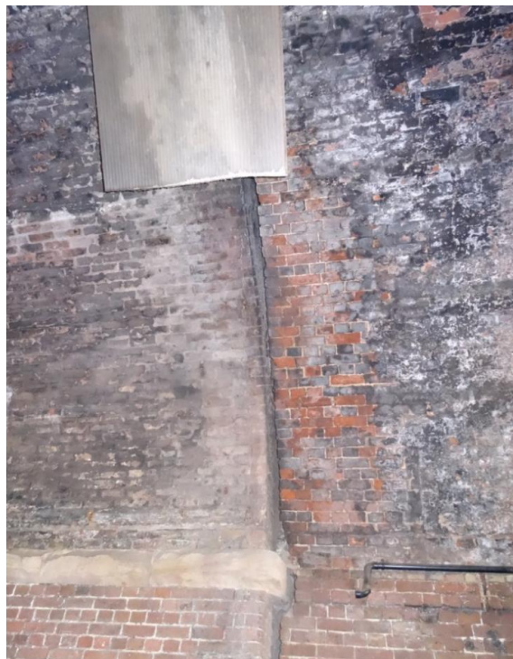
Photograph 9: Large gaps between tunnel section joins in BPZ2.
