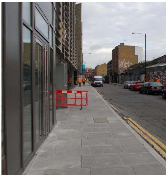
Plate 1 – View of western end of Link L5, good quality surface and effective width, albeit partially restricted with presence of construction works
