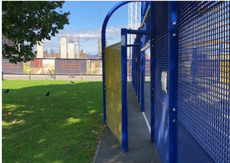
Existing entrances at goal posts - to be closed up, replaced with matching panels.
