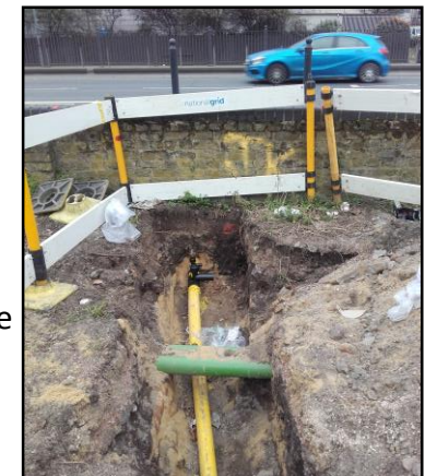
Gas pipe work in central area
