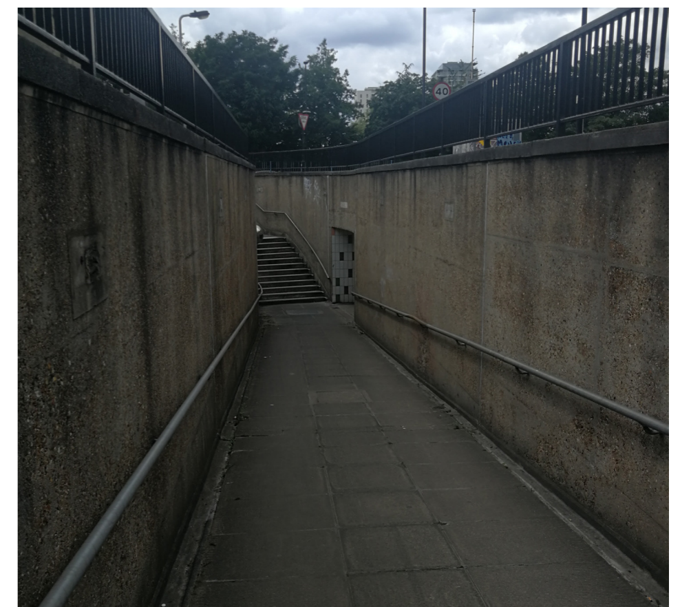
12 Fig.20 The pedestrian underpass through to Jolly's Green is in poor condition and can feel unsafe
