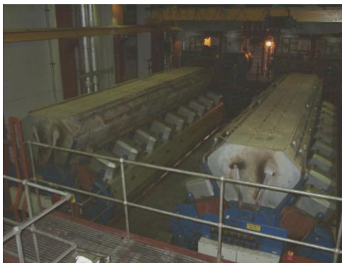
Figure 2 – Citigen CHP Engines (Photo courtesy of E.On UK Ltd)
