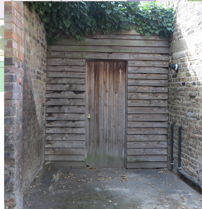
Photograph showing obstruction to shared access route
