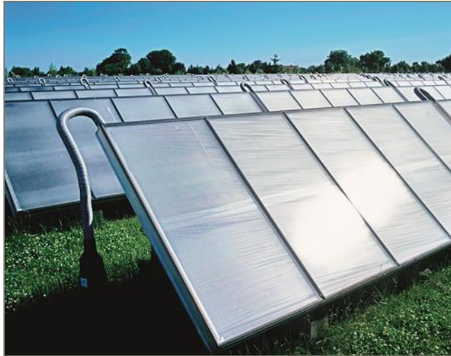
Figure 22: Photograph of Solar Thermal Array (Ramboll Image Bank Courtesy of Scanpix)
