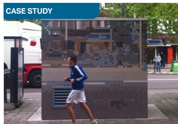
CASE STUDY FIG 6.7 Secondary distribution substation, Rotterdam, Netherlands Image credit: Emilie Chalcraft in dezeen
