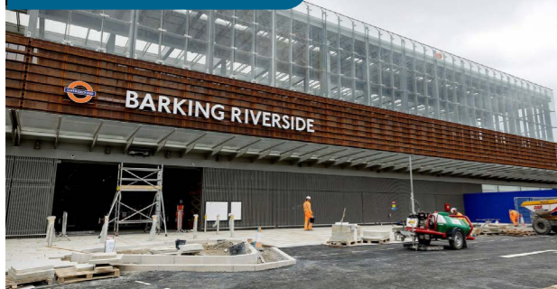
FIG 5.15 A brand-new station at the heart of Barking Riverside opened to customers in July 2022. Operating at four trains an hour, it now takes just seven minutes to travel to Barking station and connect to services to central London. Image credit: TfL
