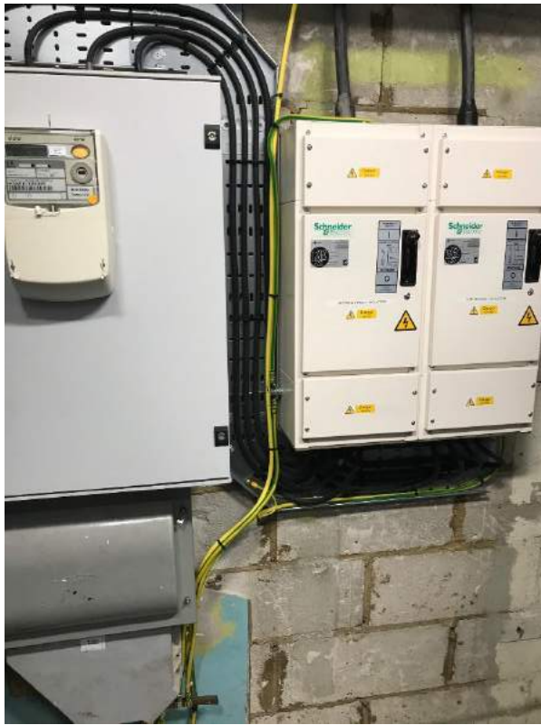
Photo 1: Onsite electrical switchroom, contained behind an area of shelving.
