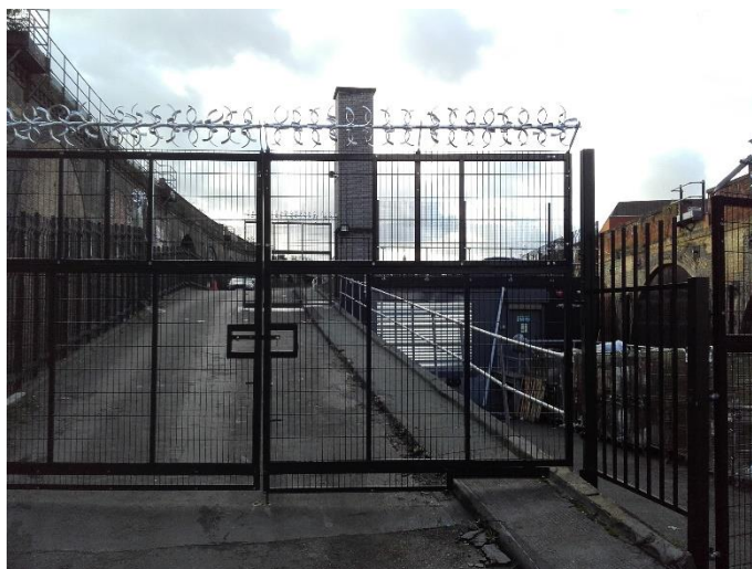
Photograph 1 Concrete ramp leading to flat roof of building B1, viewed from the east.
