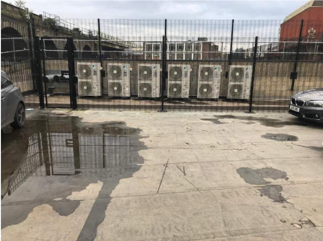
Photo 3: Air conditioning plant located within the staff carpark on the roof.
