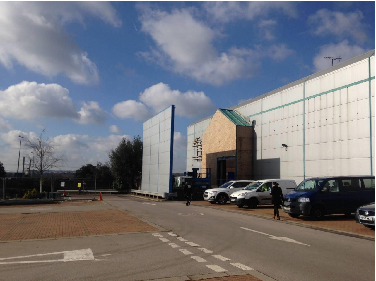
Figure 23: View west from the centre of the site towards partially demolished warehousing.
